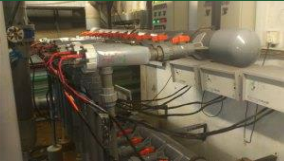
Swimming pool ionization treatment systems
