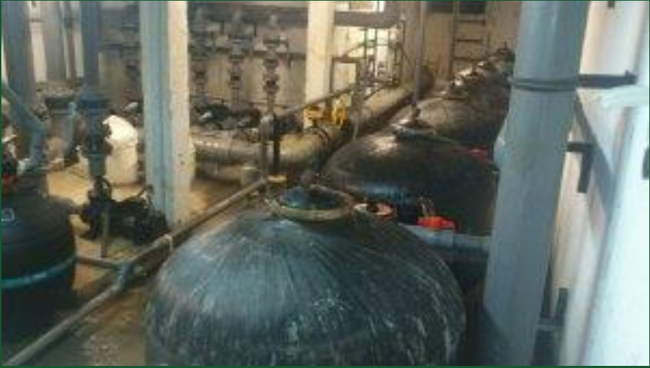
Swimming pool sand filtration Our pool does not use conventional chlorine treatment but various filtration and purification steps
